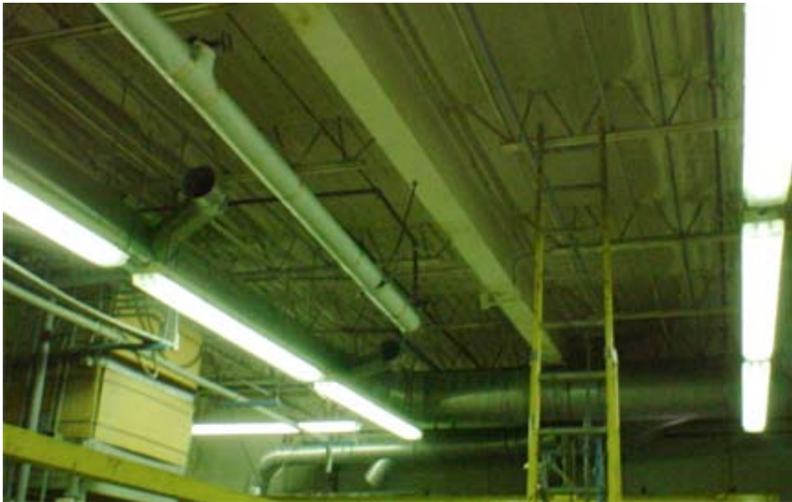
ILLUSTRATION 11: VIEW OF SECOND TEST SITE SELECTED FOR EVALUATION OF STAYFLEX™ SYSTEM AFTER 18 YEARS OF SERVICE.
