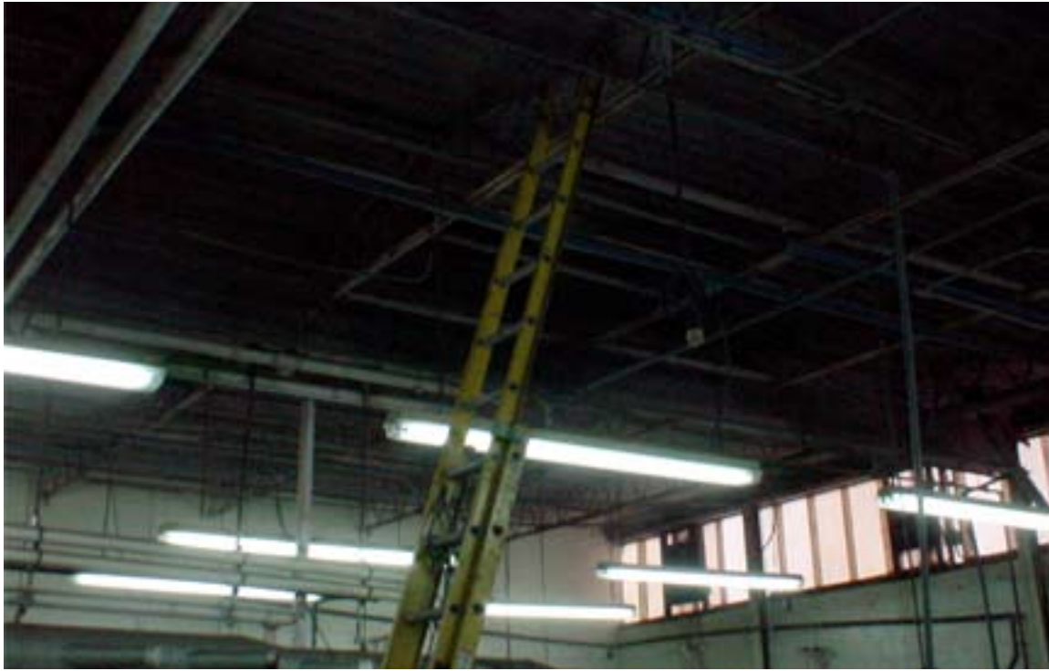
ILLUSTRATION 1: GENERAL VIEW OF TEST SITE SELECTED FOR EVALUATION OF STAYFLEX™ SYSTEM AFTER 18 YEARS OF SERVICE.
