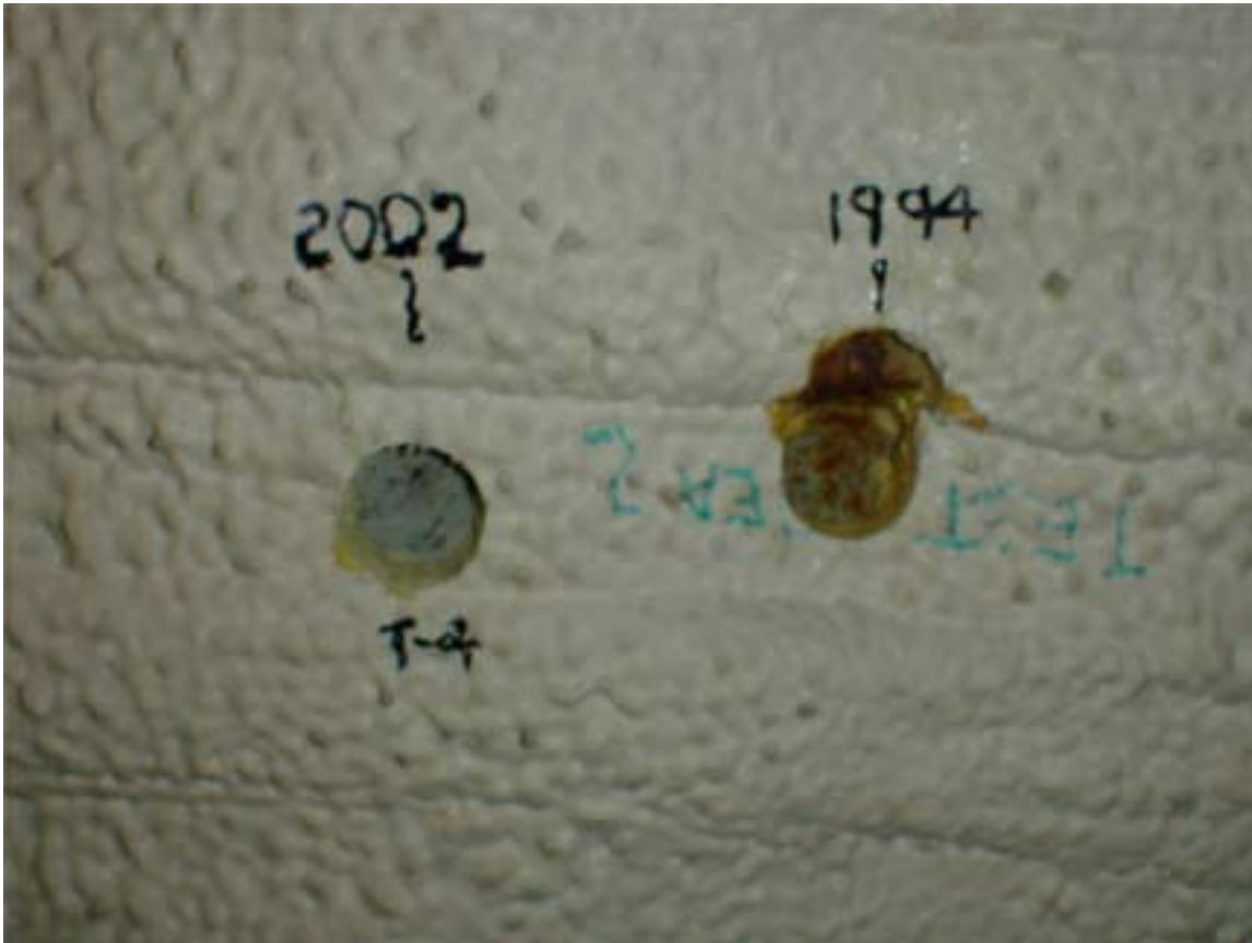
ILLUSTRATION 14: CORE SAMPLE 4 WAS TAKEN IN PROXIMITY TO A 1994 TEST REGION FOR COMPARISON PURPOSES. A SLIGHT INCREASE IN THE NUMBER OF PINPOINT CORROSION CELLS WAS NOTED IN THE 2002 TEST LOCATION. THE EXPOSED TEST LOCATION FROM 1994 HAS DRAMATIC SECTION LOSS IN EXCESS OF 50%. THIS WOULD SUPPORT THE SUPERIOR PERFORMANCE OF THE STAYFLEX™ SYSTEM OVER THE PAST 18 YEARS.
