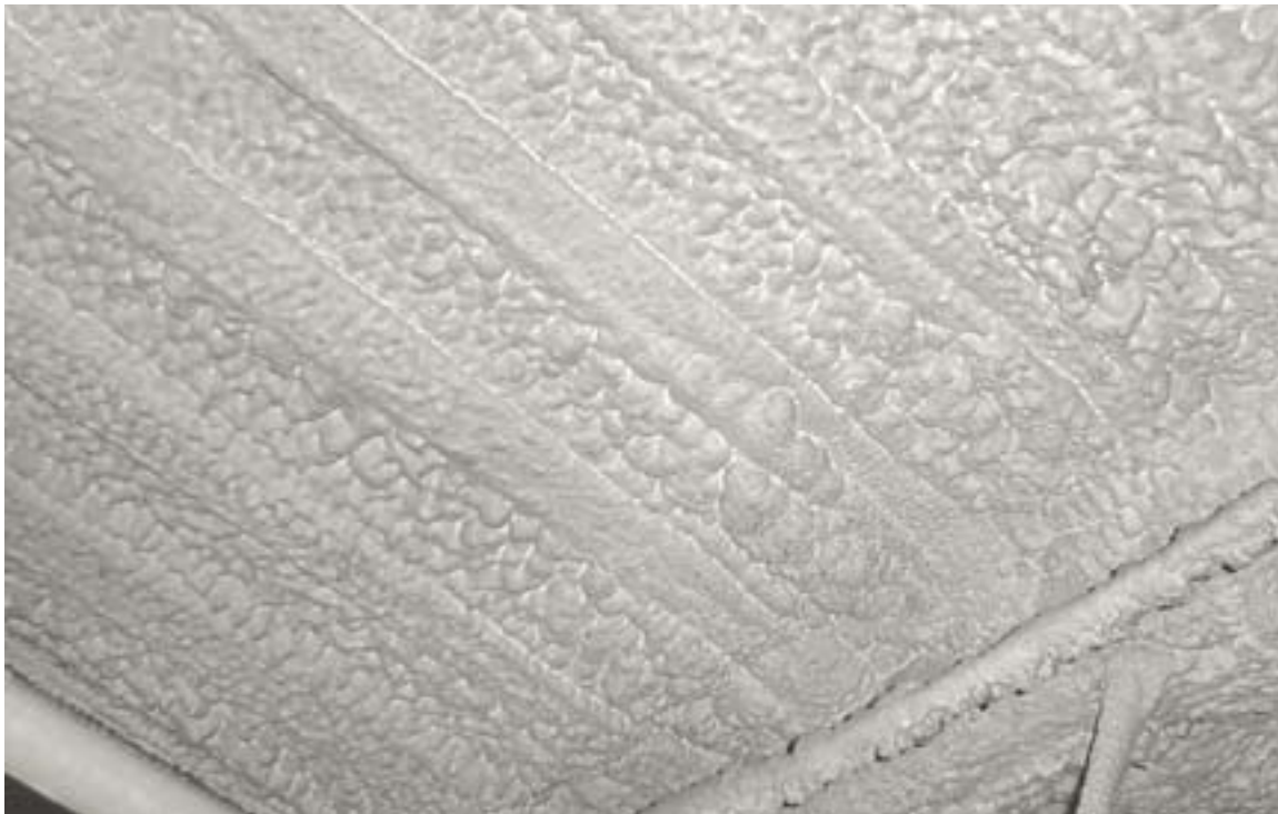
ILLUSTRATION 2: GENERAL VIEW OF STAYFLEX™ SYSTEM IN SERVICE IN A HIGH ACID VAPOR ENVIRONMENT AFTER 18 YEARS. NO EVIDENCE OF DELAMINATION OR SAGGING DISCOVERED.
