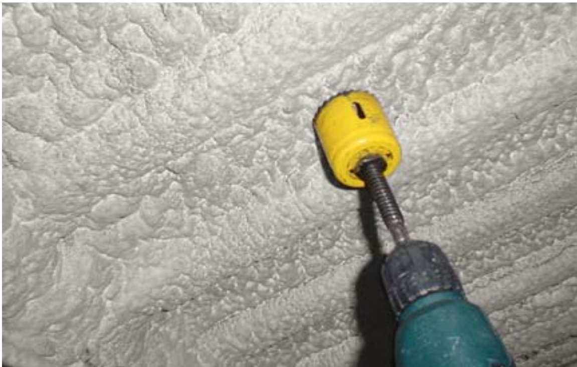
ILLUSTRATION 4: VIEW OF CORE SAMPLING EXTRACTION FOR SUBSURFACE EVALUATION.
